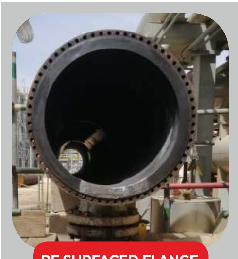
RE SURFACED FLANGE
